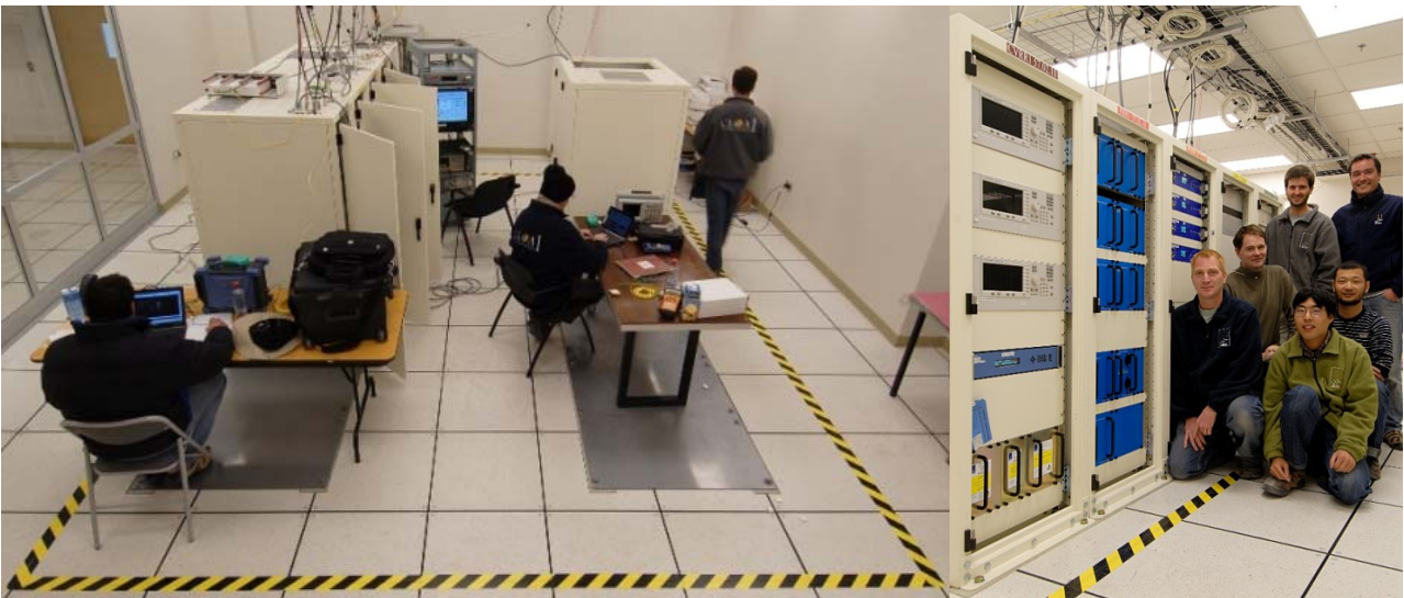
Figure 6. Installation and testing of the central local oscillator system at the AOS Technical Building
