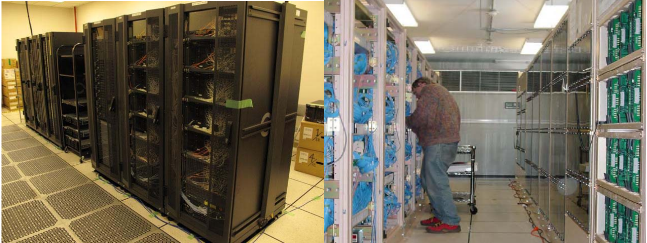
Figure 7. The ACA correlator and the 64-input correlator (two quadrants visible) installed at the AOS Technical Building
